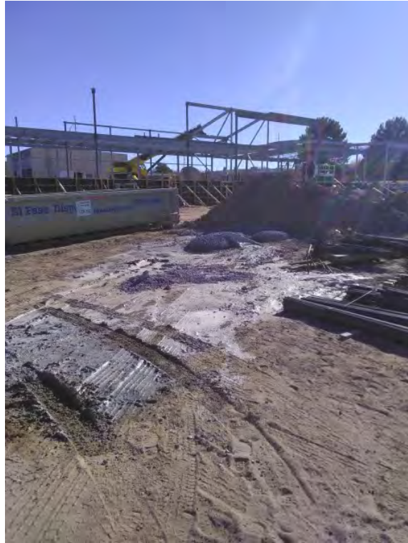
Site Walk Deficiency Photos - Concrete washout on ground NW corner of structure
