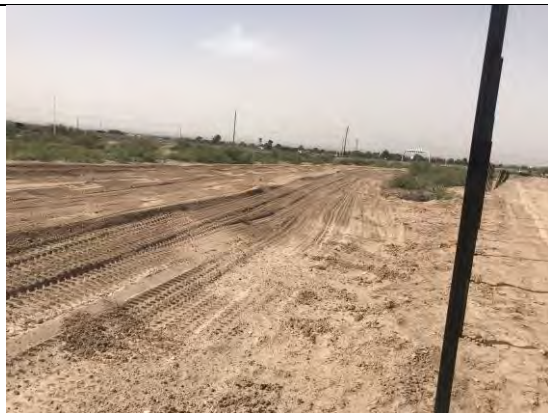
View of drainage swale 3. Swale has been regarded. Earth berm No. 9 removed, and permanent drainage measures installed.
