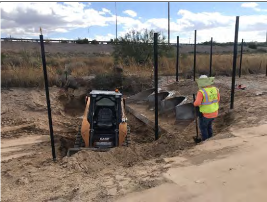
View of drainage swale No. 4. Crew removing dirt for installation of rock on upstream entrance.
