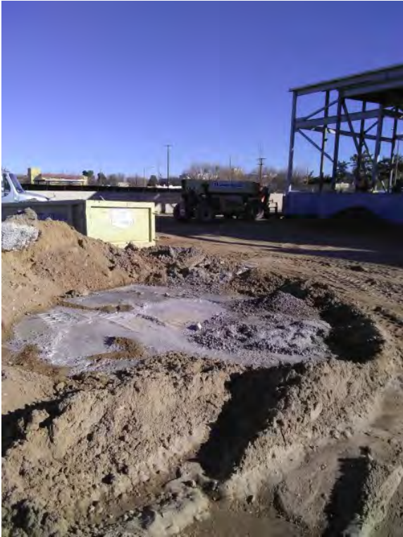
Site Walk Deficiency Photos - Unlined washout pit NW
