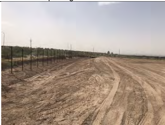
View of drainage swale No. 4. Adjacent earth berm removed, and permanent drainage measure installed.
