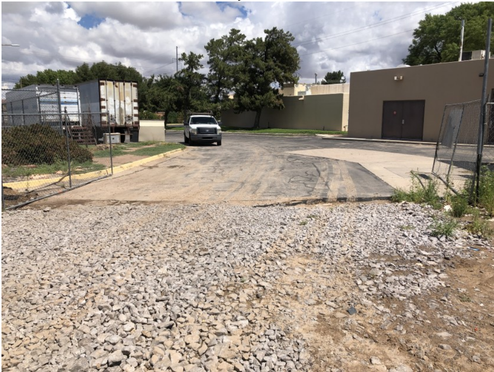
Site Walk Deficiency Photos - NE entrance
