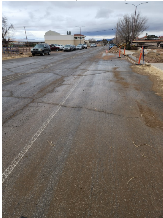
Site Walk Deficiency Photos - Sweep Street
