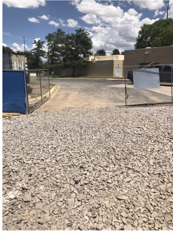
Site Walk Deficiency Photos - NE entrance
