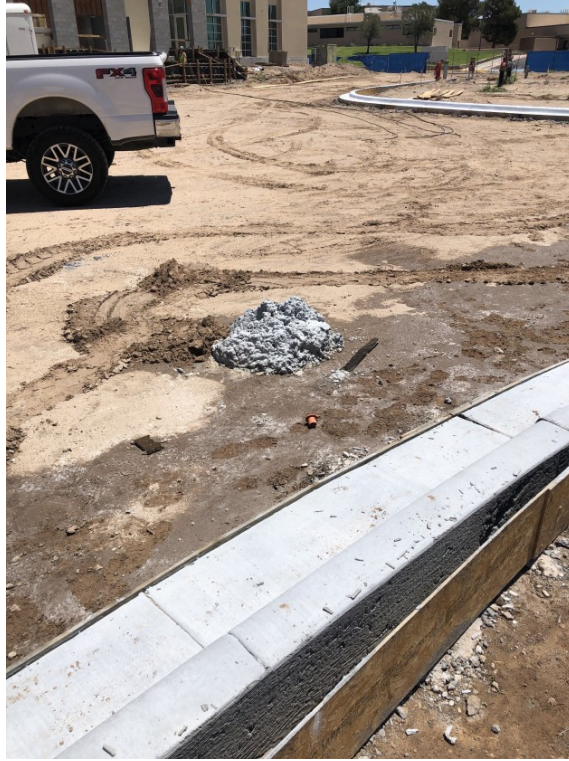
Site Walk Deficiency Photos - NW corner Concrete washout on ground
