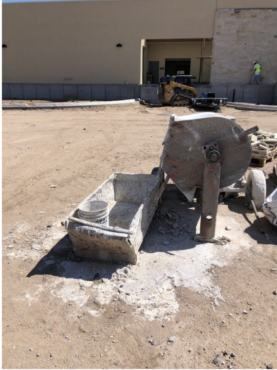
Site Walk Deficiency Photos - Mortar washout NW
