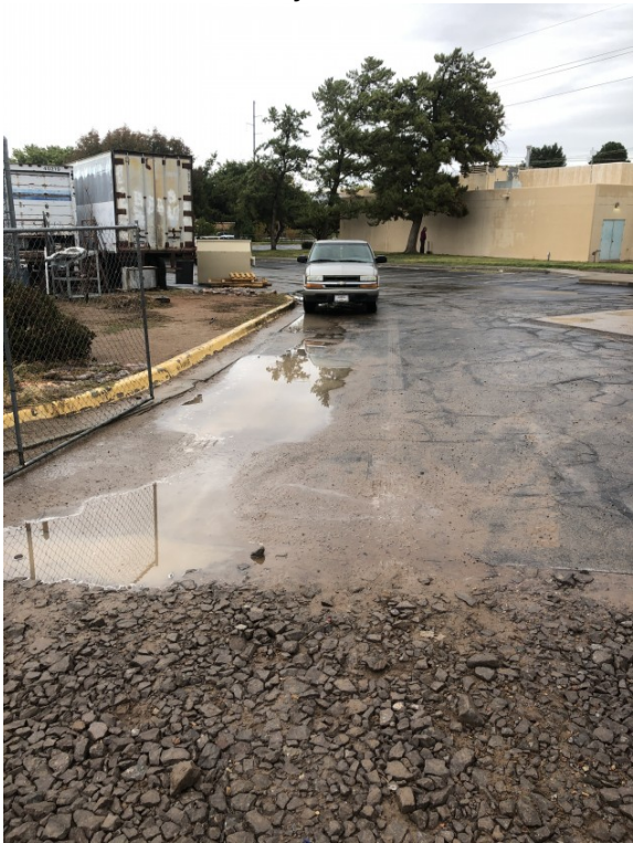
Site Walk Deficiency Photos - NE entrance
