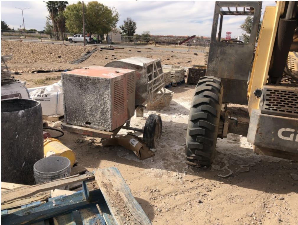
Site Walk Deficiency Photos - Mortar Mixer Area
