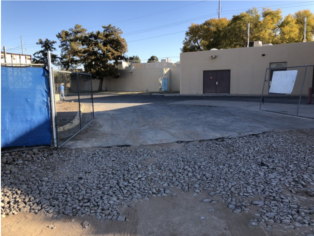
Site Walk Deficiency Photos - NE entrance
