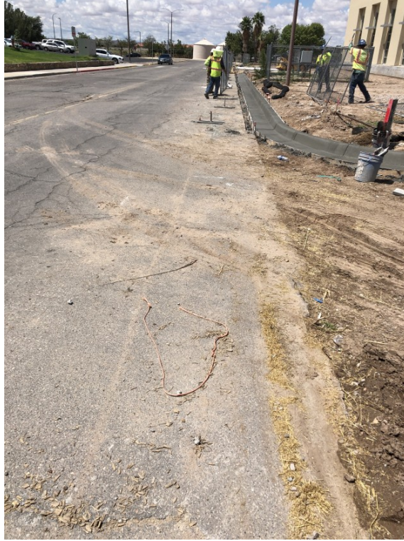
Site Walk Deficiency Photos - Sweep Sediment on Greg St.
