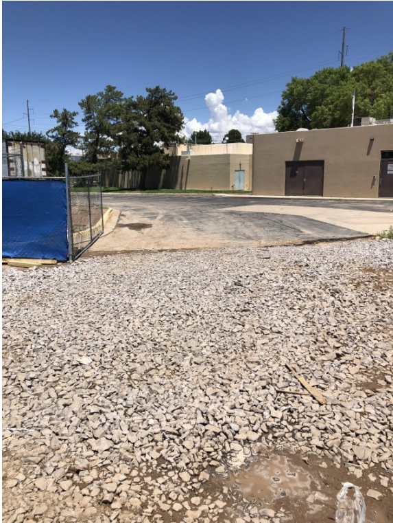
Site Walk Deficiency Photos - NE entrance
