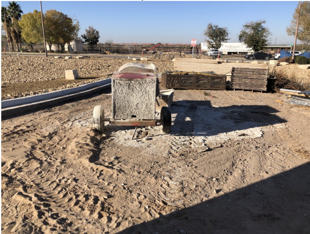
Site Walk Deficiency Photos - Mortar Mixer Area
