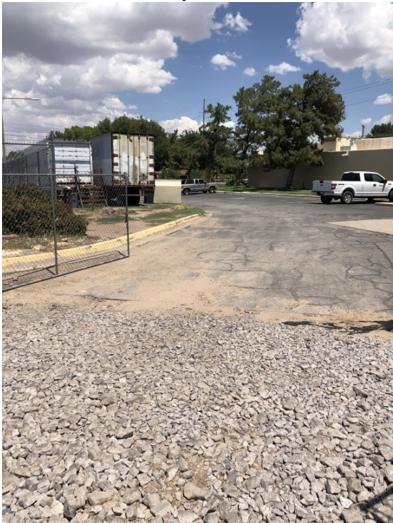
Site Walk Deficiency Photos - NE entrance
