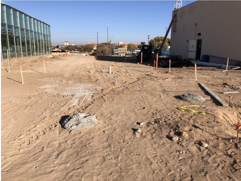
Site Walk Deficiency Photos - SE Concrete Washout
