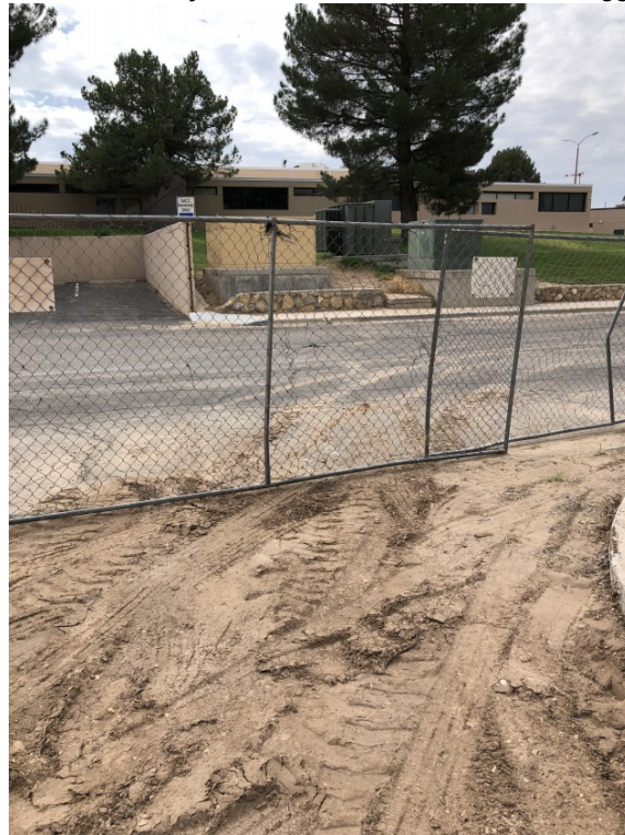
Site Walk Deficiency Photos - South entrance onto Gregg St.
