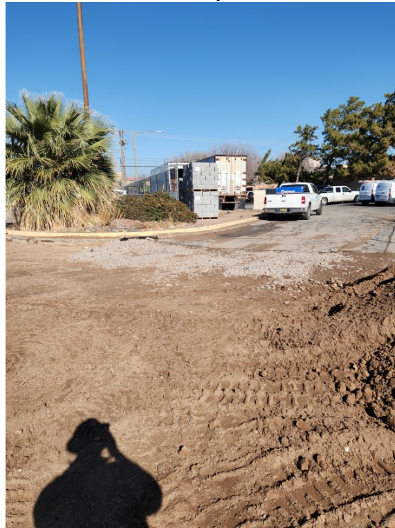
Site Walk Deficiency Photos - VTC
