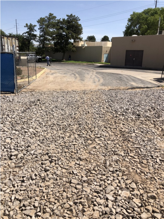
Site Walk Deficiency Photos - NE entrance
