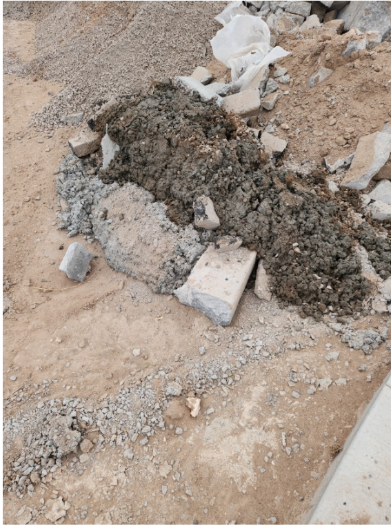
Site Walk Deficiency Photos - Concrete Spill
