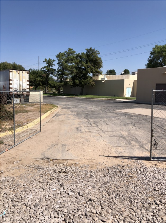
Site Walk Deficiency Photos - NE entrance
