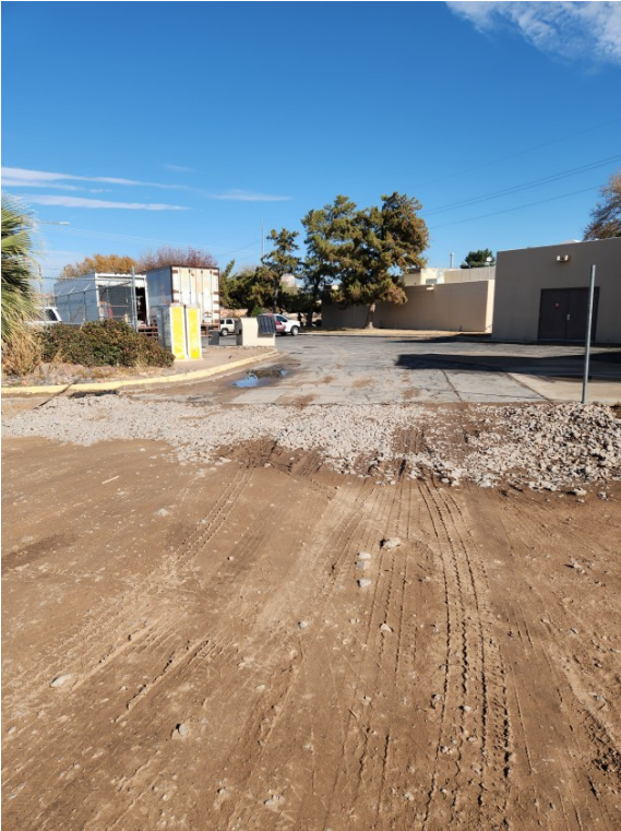
Site Walk Deficiency Photos - NE entrance
