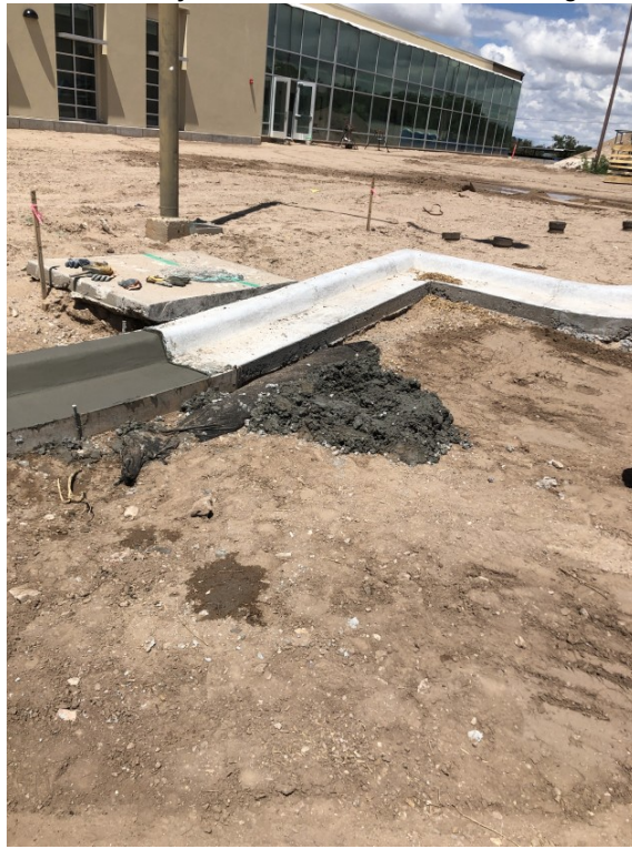
Site Walk Deficiency Photos - Concrete washout on ground SE
