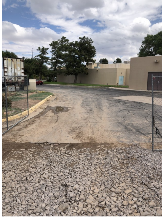
Site Walk Deficiency Photos - NE entrance
