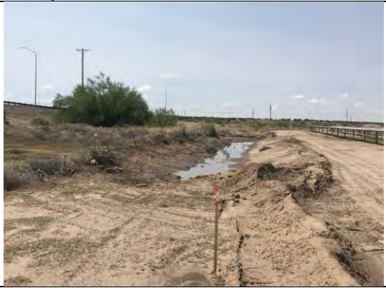
View of drainage swale No. 4 on east side of site. Water entering project site has been detained.
