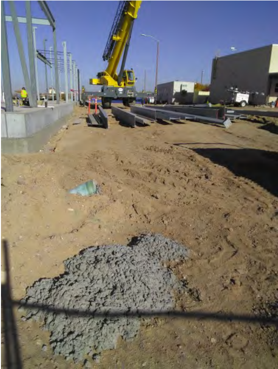
Site Walk Deficiency Photos - Concrete washout on ground SE corner of structure
