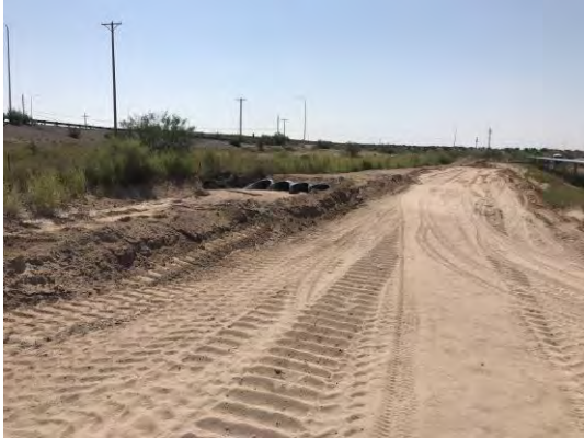
View of drainage swale No. 4. Berm has been built up on west edge of berm.
