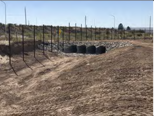
View of rock protection installed around drainage pipe outlet in drainage swale 3.
