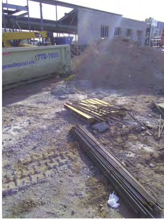
Site Walk Deficiency Photos - Concrete washout on ground NW corner of structure
