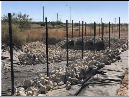
View of rock placement on top of plastic barrier in drainage swale No. 4.
