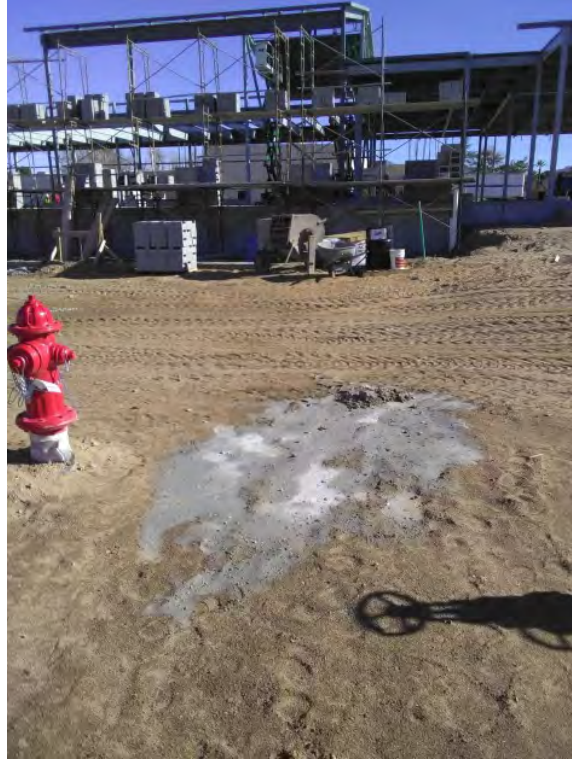
Site Walk Deficiency Photos - Concrete washout on ground SW corner of structure
