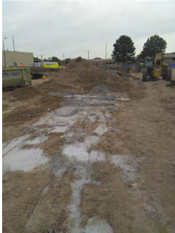
Site Walk Deficiency Photos - Concrete washout on ground NW corner of structure
