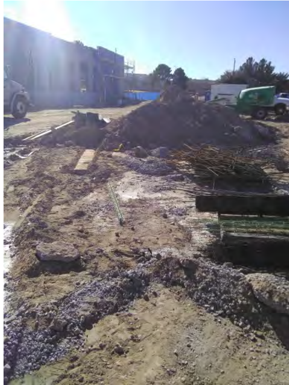
Site Walk Deficiency Photos - Concrete washout on ground NW corner of structure
