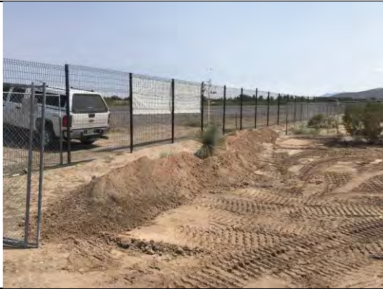
View of earth berm No. 2 that has been extended to meet rock driveway entrance.
