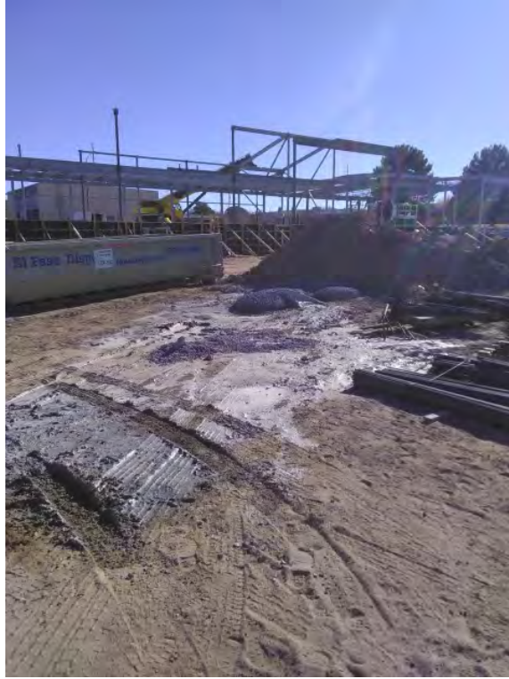
Site Walk Deficiency Photos - Concrete washout on ground NW corner of structure
