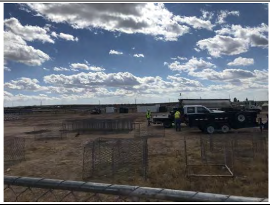
View of crew placing rock in wire basket for installation in drainage swales. .
